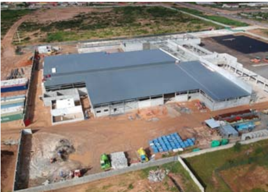
A new Shoprite store under construction in Luena, Moxico province, Angola. Shoprite is the biggest retailer in Africa.
